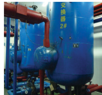
Pict.37 Hot water storage tank
