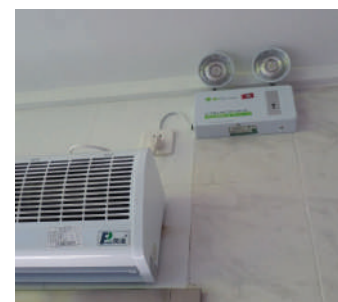
Pict.33 Security lighting
