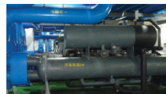
Pict.38 Screw compressors (new technical supply)
