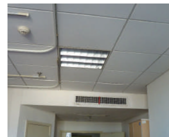
Pict.22 Acoustic ceiling patientroom
