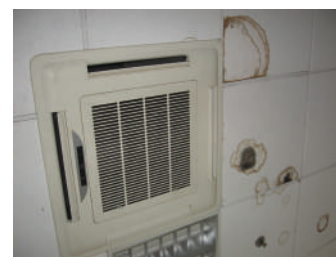
Pict.41 Moisture damages due to condensation from cooled supply air (new construction)
