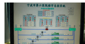
Pict.48 Central building control system - technical supply
