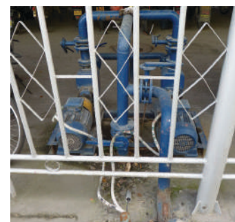
Pict.52 Pump station water supply
