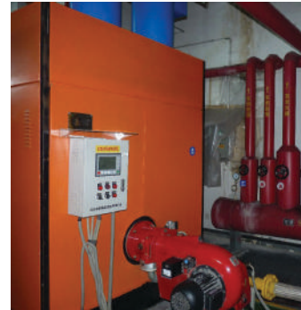
Pict.36 Heating system - solid fuel boiler (new technical supply)
