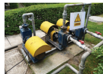
Pict.51 Pump station water supply
